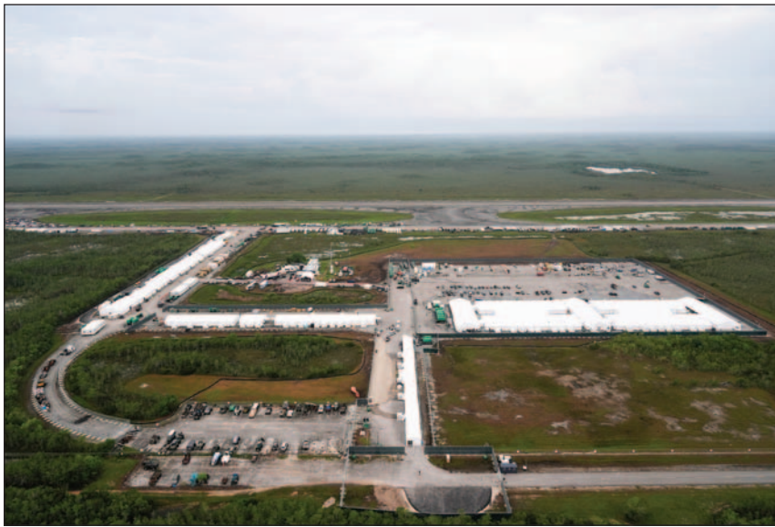
Work progresses on a new migrant detention facility dubbed “Alligator Alcatraz,” at Dade-Collier Training and Transition facility in the Florida Everglades, on July 4 in Ochopee, Fla. (AP Photo)
